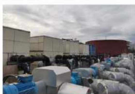
Chiller Plant 冷水機房
